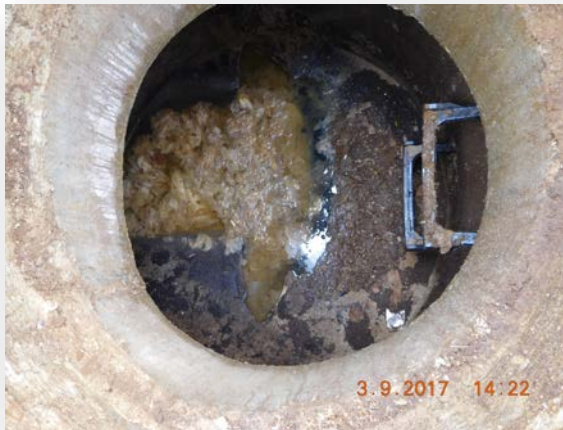
City sanitary sewer manhole
