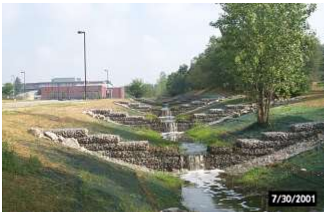
Victor Parkway Storm Drain
